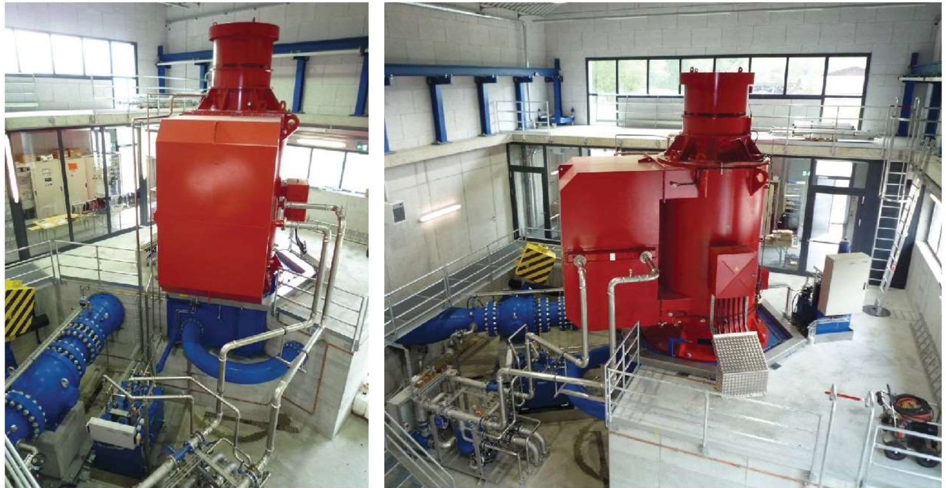
Figure 12-11: Photo of Similar Sized Pelton Wheel Generator Installation
